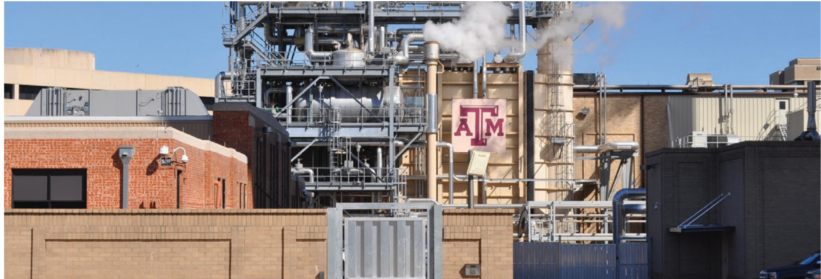
The Central Utility Plant at Texas A&M University provides power across campus.
