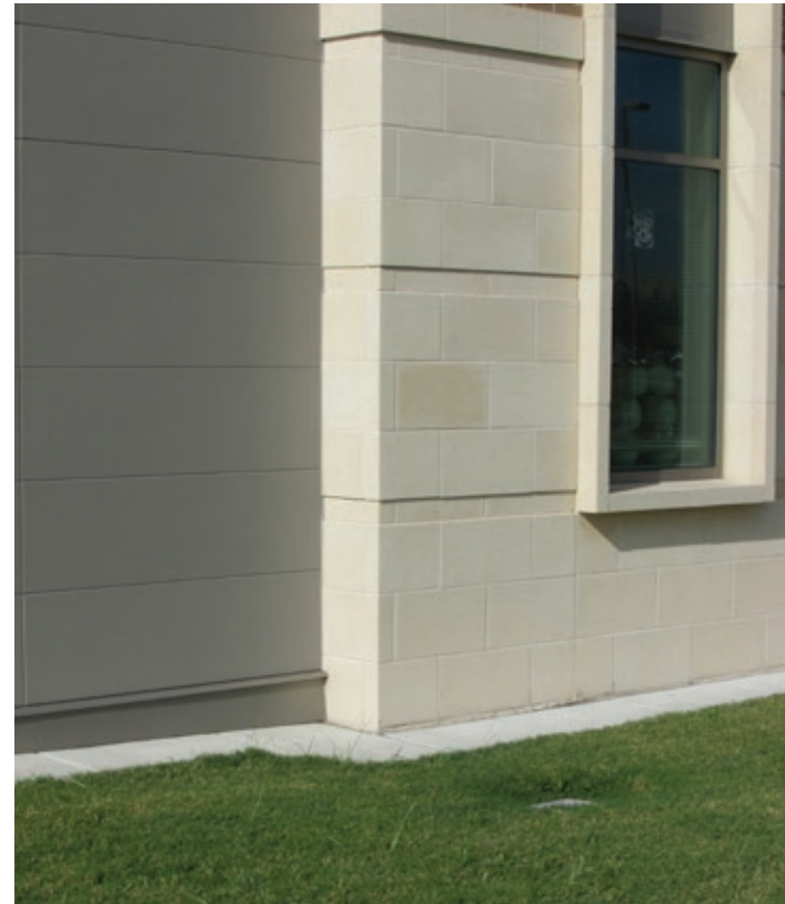
Limestone Cladding and Window Surround at the Physical Education Activity Program Building
