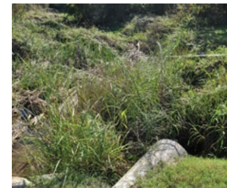
Erosion at White Creek
